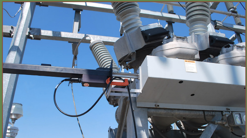
25" transducer on Siemens SPS2 Breaker
