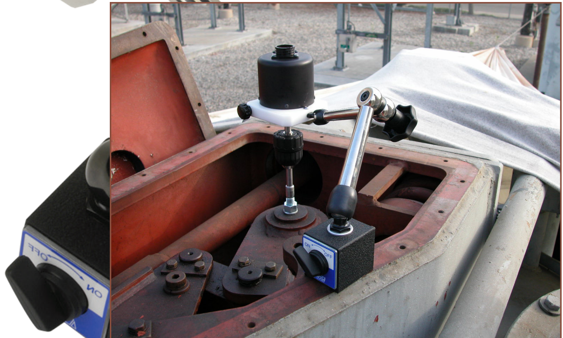
Type 3 rotary transducer on a Federal Pacific breaker
